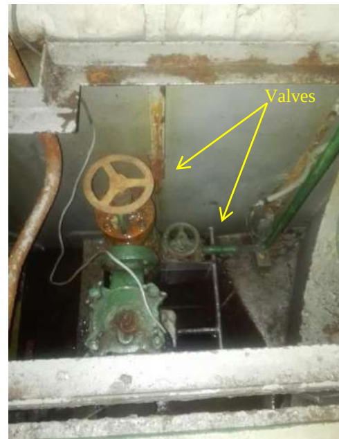
Figure 1: Bad valve placement in OPV-A
